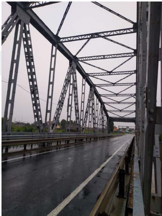
Bridge over the Neman River at the 65,774 km of the P-41 road
